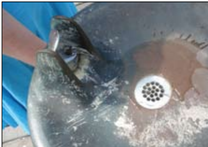
Drinking Fountains performed poorly this year due to lack of pressure, leaks, and broken spigots.
