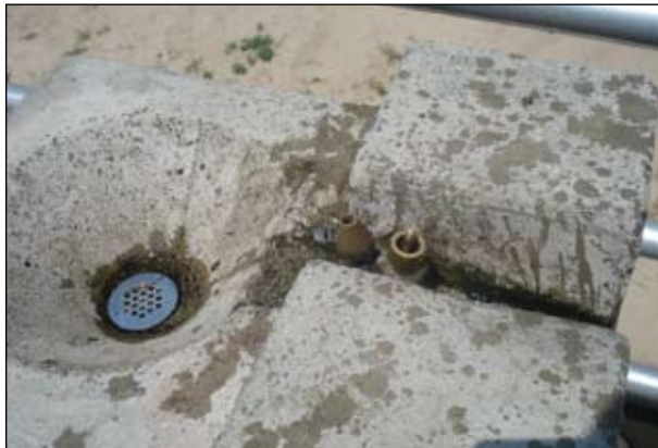
This Drinking Fountain at Rockaway Beach is missing a critical part.
