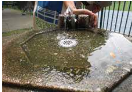
Drinking fountains with standing water are automatically failed.
